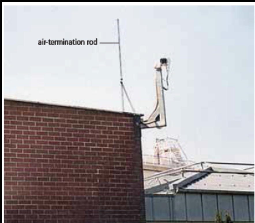
Fig. 9.7.2 Camera for video surveillance in the protective area of the air-termination rod
